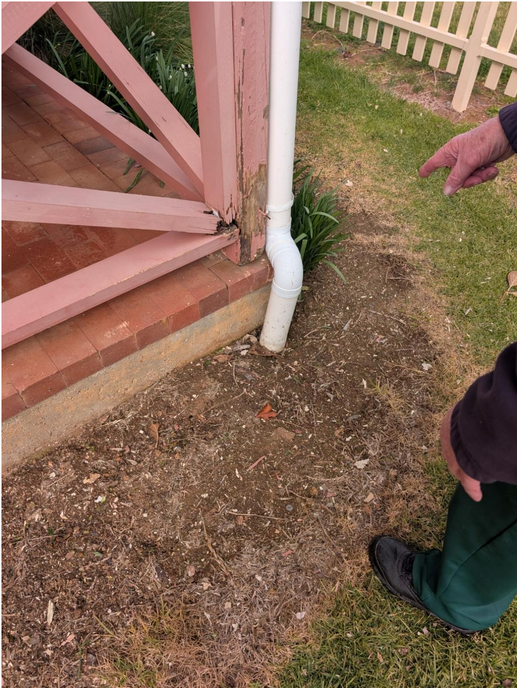
Location: Verandah, adjacent to main entry door to Bradman Museum cottage. It was reported that there may be a blockage or damage in this pipe, which should channel rainwater to the gutter on Adams St. Volunteers found significant pooling in recent rains.
