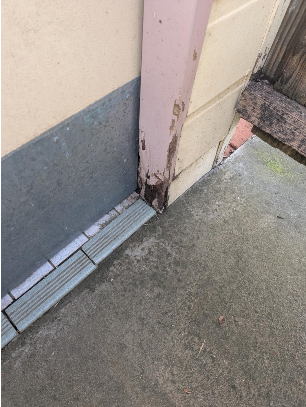
Location: Entry door to male toilets – door is now permanently locked as the timber rot has resulted in the lower hinge coming off.
