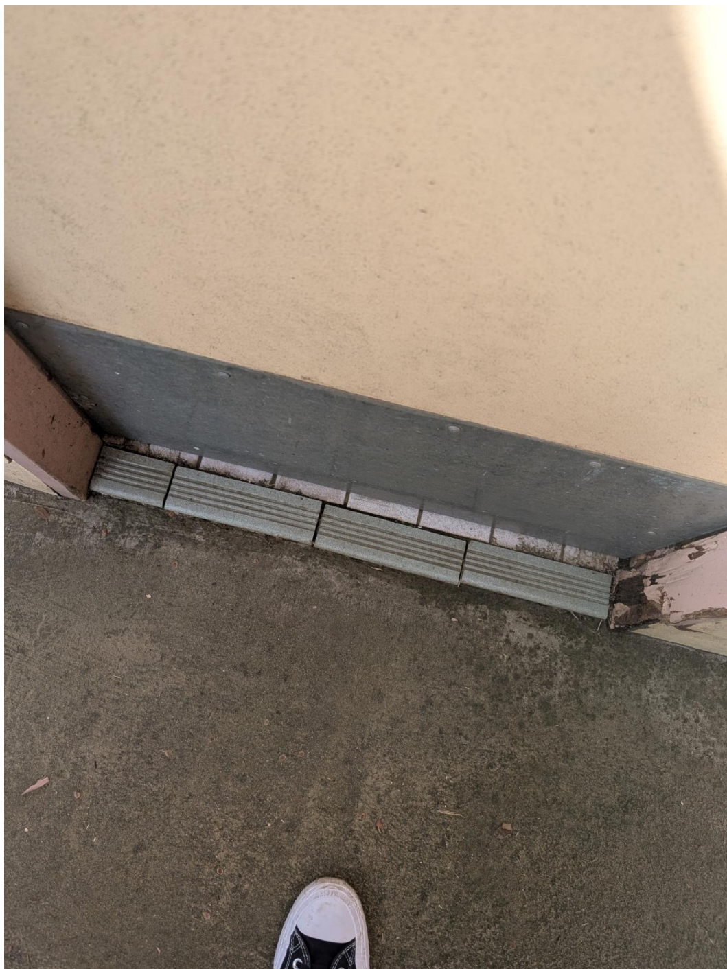
Location: Entry door to male toilets – door is now permanently locked as the timber rot has resulted in the lower hinge coming off. Some loose tiles.
