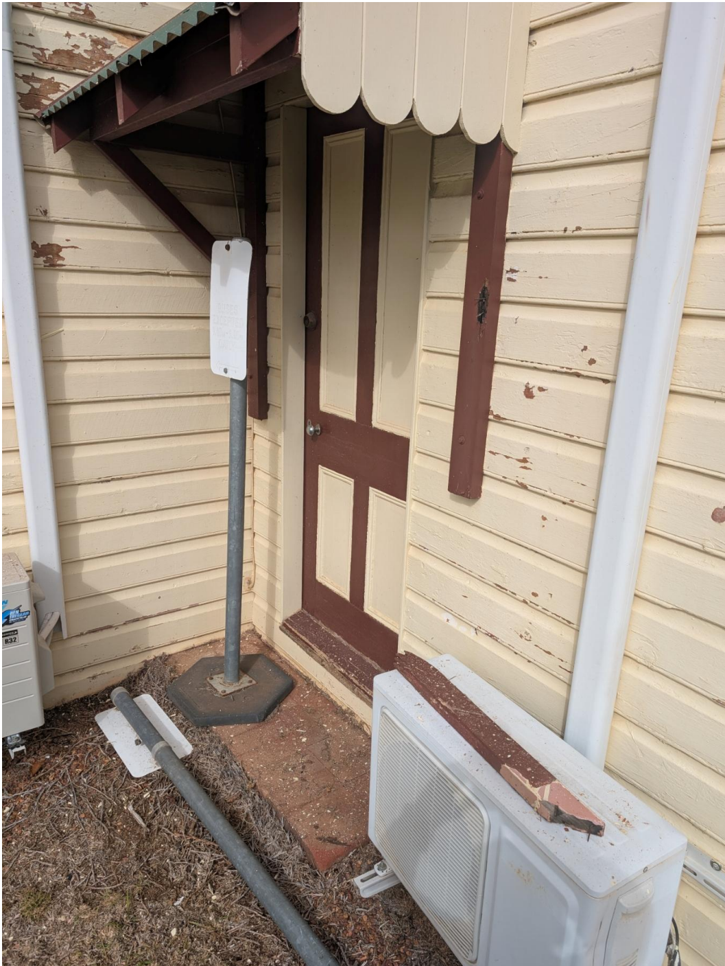
Location: Rear of Bradman Museum cottage, support arm on awning has rotted off
