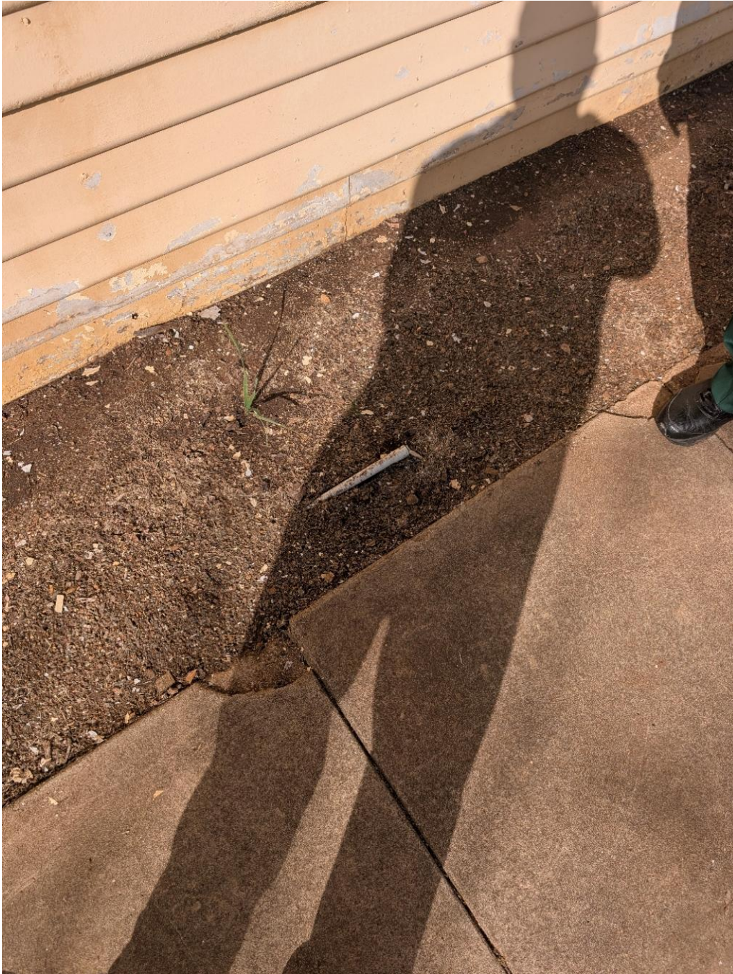
Location: Path next to memorabilia cottage – electrical wire and conduit exposed.
